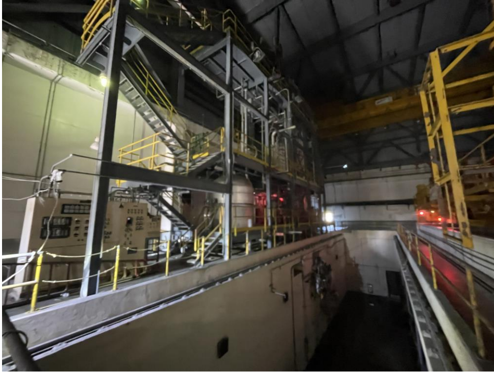
Cask washpit service equipment platform
