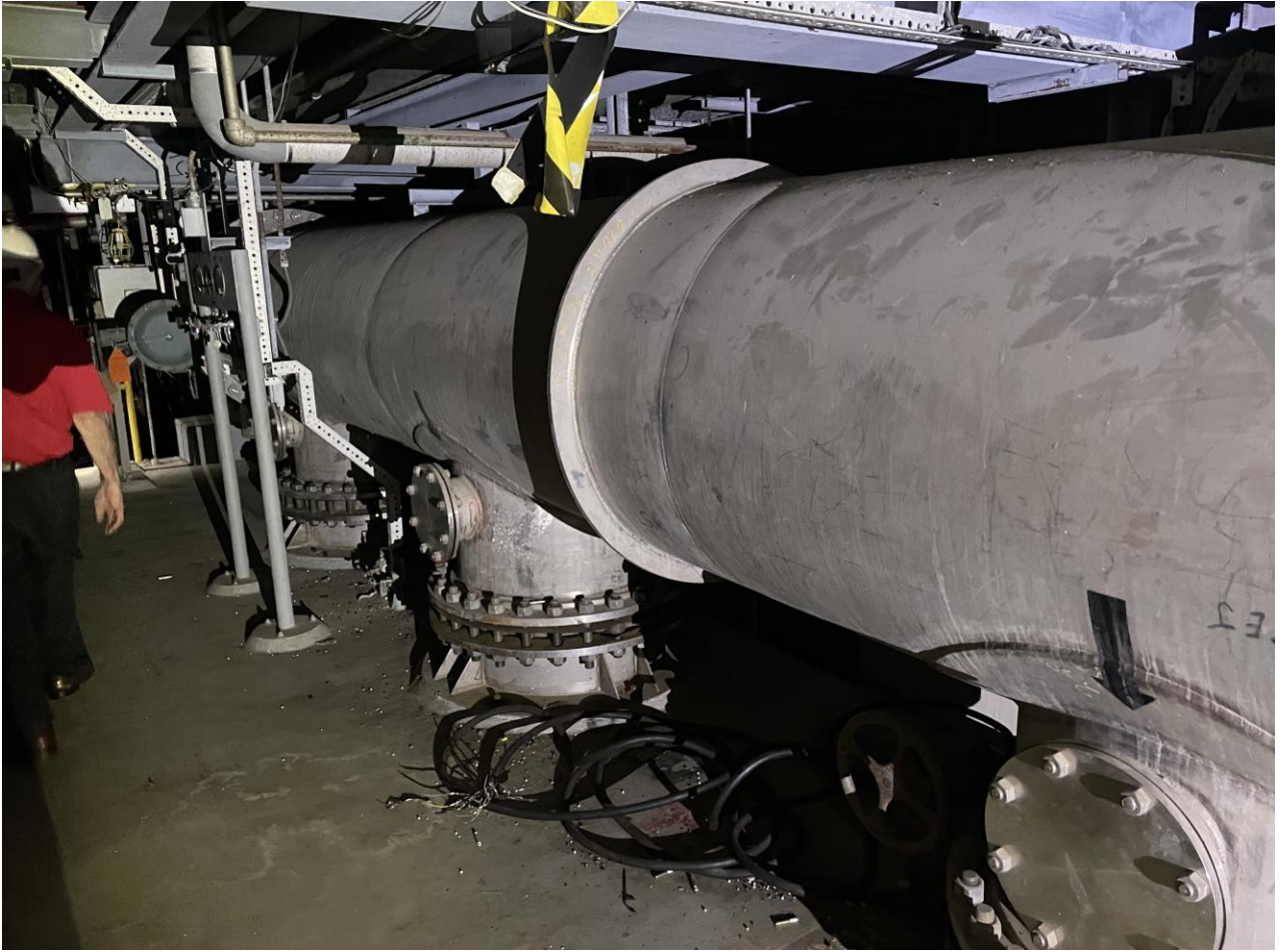
Stainless steel air filter ductwork in basement
