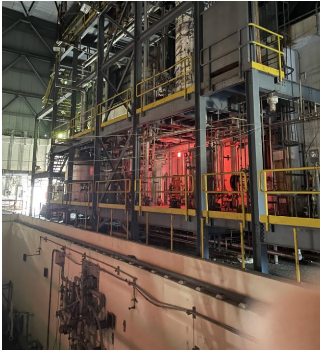
Cask wash basin support equipment
