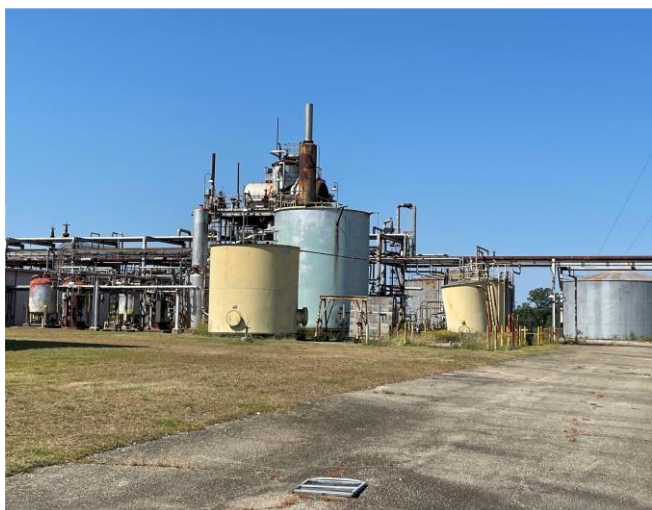
Facility tank farm
